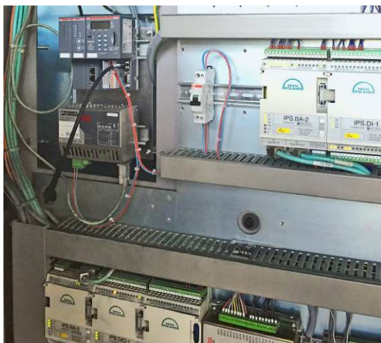
ABB controls in operation alongside PECOM units in Bordeaux
