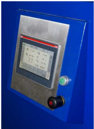
ABB control panel on the Wifag OF370 in Halifax
