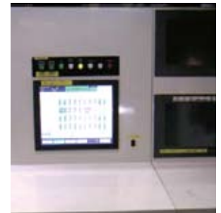
The automatic controls can be tracked in real time on the touch screen of the operator console.
